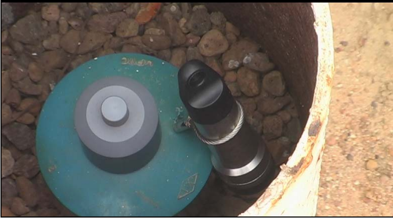
Figure 19: Baro Diver placed inside the housing structure of the bore. Note the secure attachment of the steel cable to the bore cap
